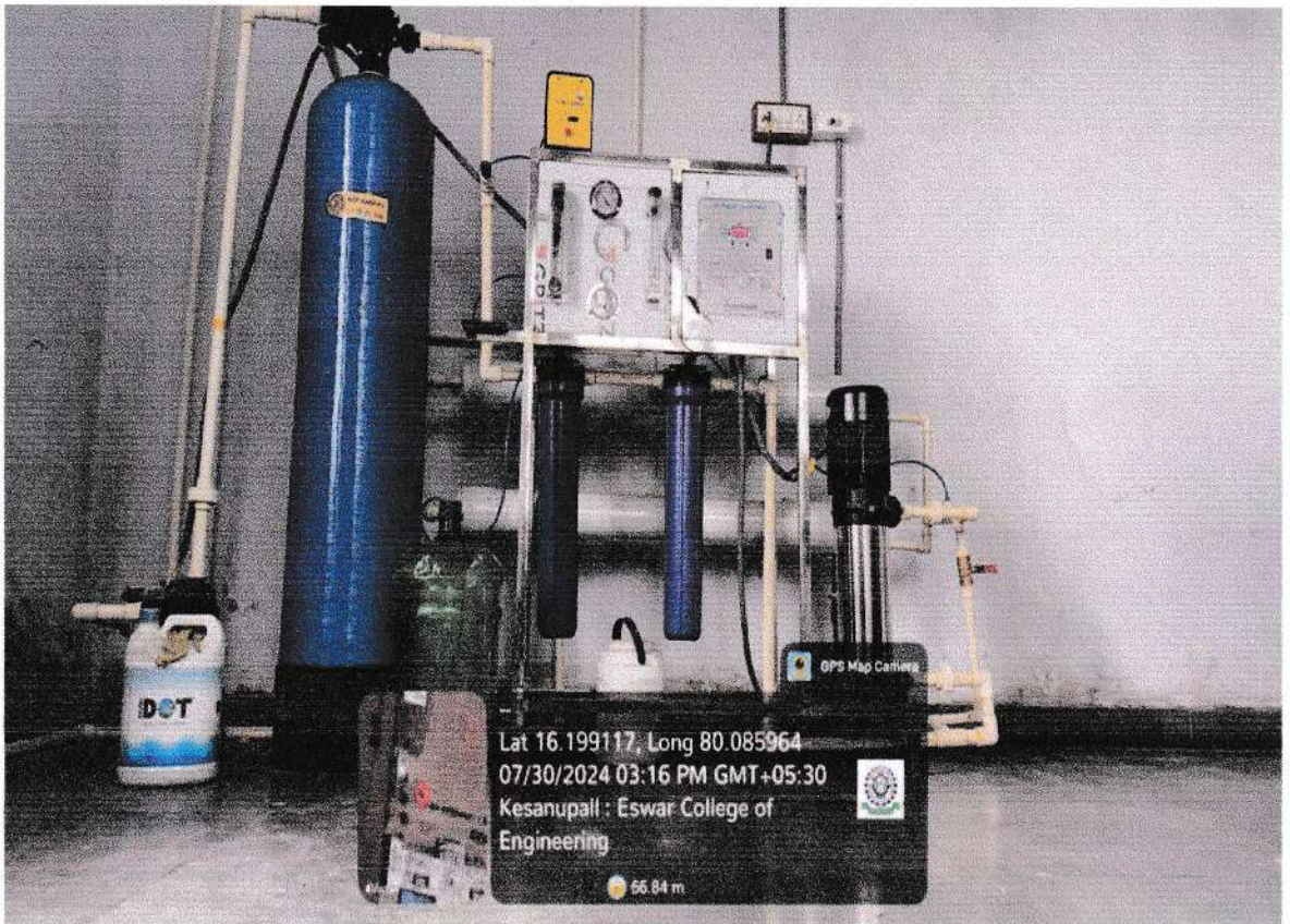
Reverse Osmosis Water Treatment Plant
